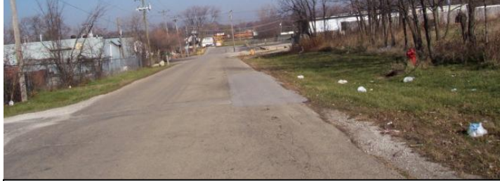
Lack of Sidewalks on Crane Street in Aurora Township.
